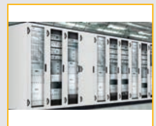
Signalling & Passenger information systems
